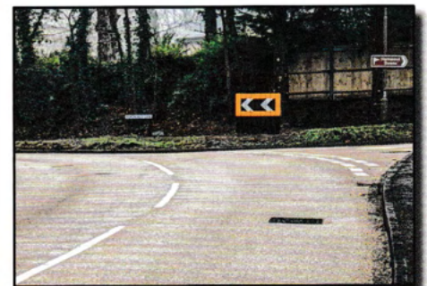
New 'slow' signs and corner warning signs (above) and anti-skid surfaces and new chevrons on Cokes/Nightingales corner (right)
